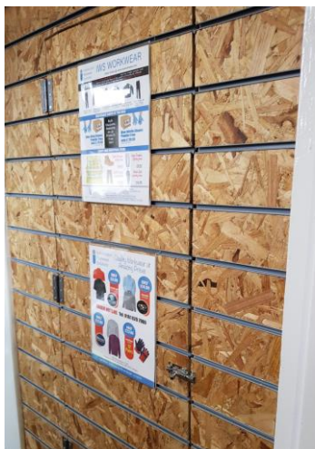
Door leading to Alarm Panel
