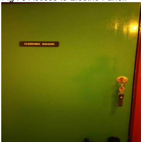
Fig . 3 Access to Electric Panel.
