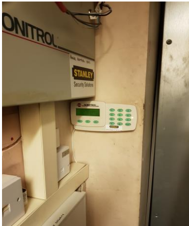
Fig 3 - Alarm Panel Location
